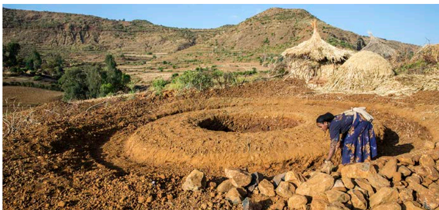
The rainwater infiltration pit is still brand new. But the prospects for vegetables are good.
